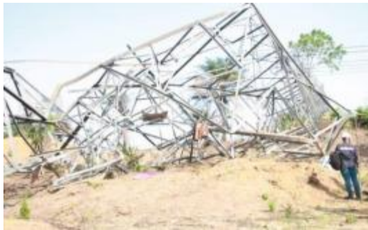
Figure 6. Vandalization of high voltage power line.
