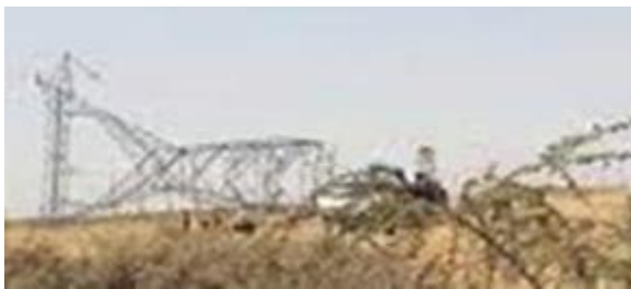
Figure 7. Vandalization of high voltage power line.
