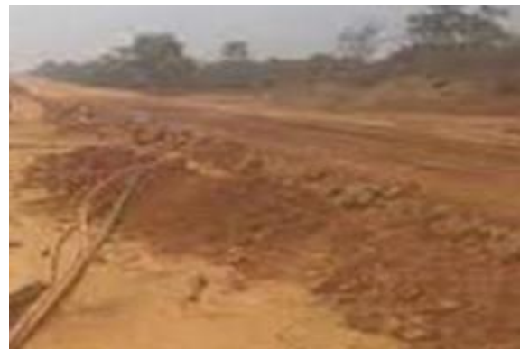
Figure 5. Vulnerable opticfibre cables during road construction.
