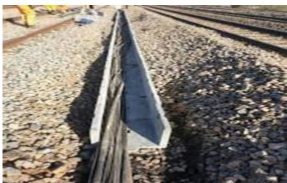
Figure 15. Telecommunication Corridor along Rail Tracks.
