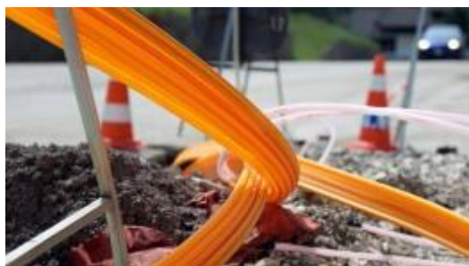
Figure 8. Vulnerable optic fibre cable deployment along road corridor.
