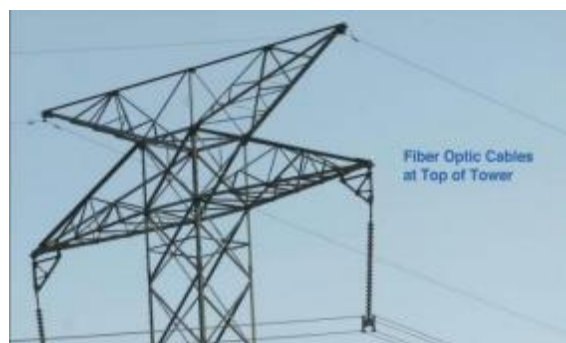
Figure 16. Telecommunication Corridor over High Power Tower Mast.
