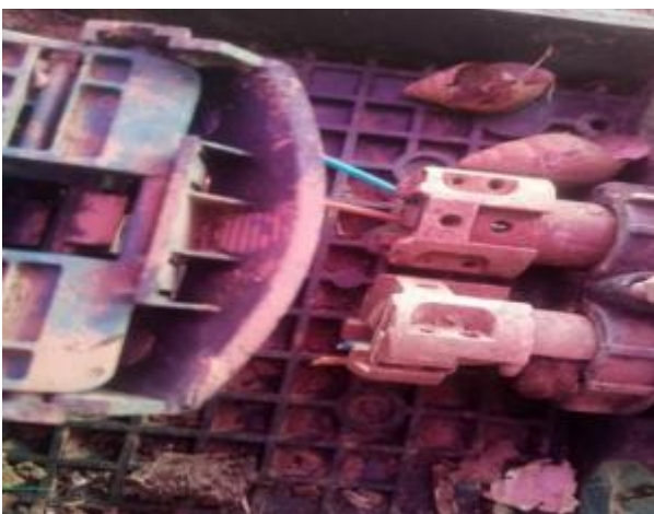
Figure 12. Optic fibre cable buffer eaten by rodents along Abuja Airport Highway Road.
